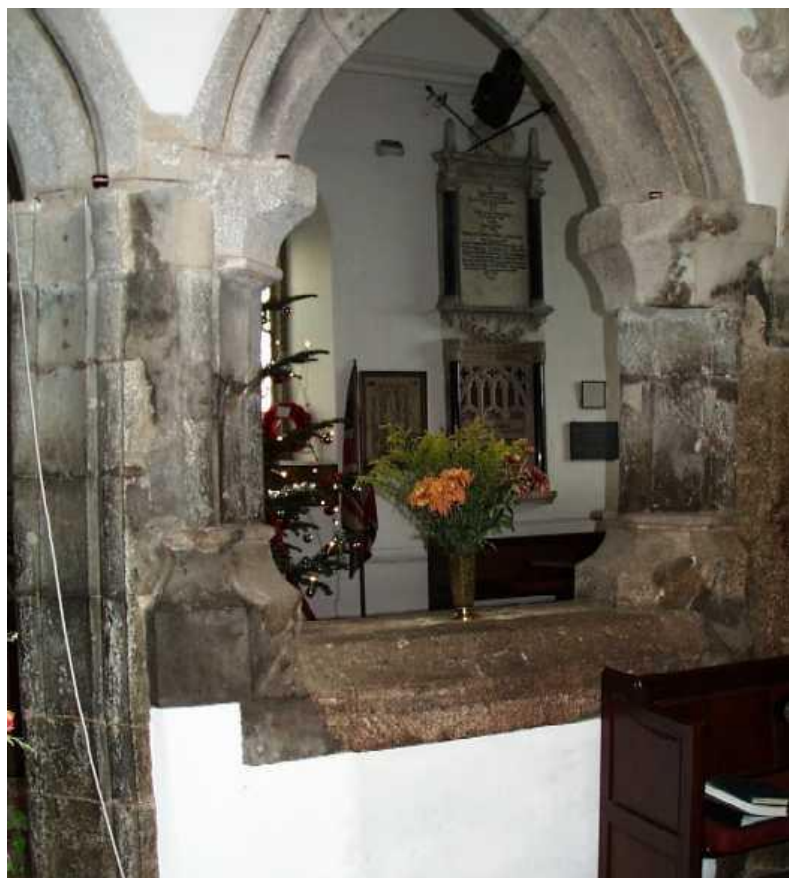
Scorched pillars and arch damaged by the fire on 23 rd July 1595.
