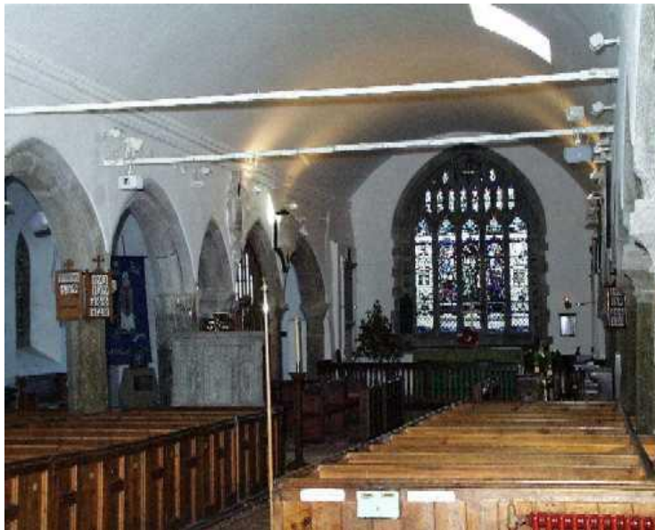
The arches on either side of the nave lean outward and further movement is prevented by unsightly tie-bars.
